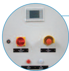
Electrical control panels
